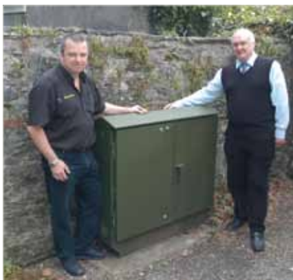
John and a local business owner next to a BT cabinet in Tavistock North
